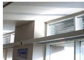
Daylight Redirecting Blinds (Daylighting Zone)
